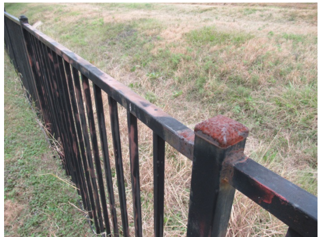
Rust and deterioration
