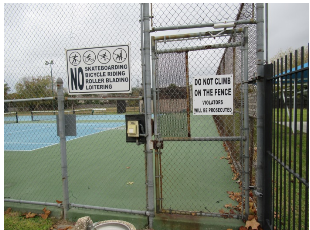
Gate rust and deterioration
