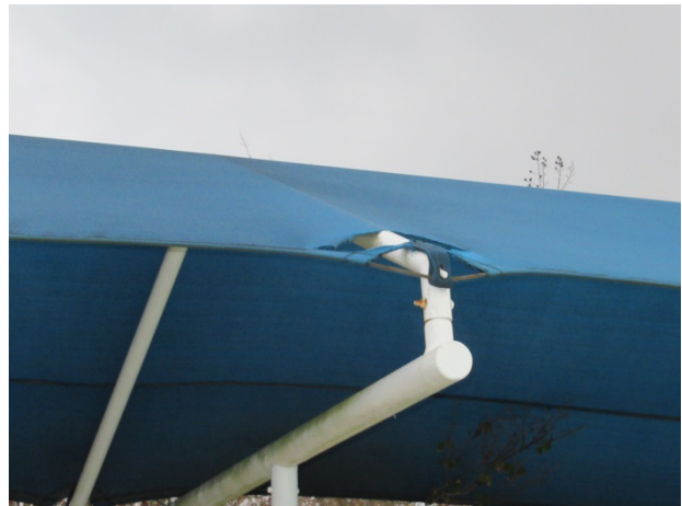
Deteriorated canvas (Replace through operating budget)
