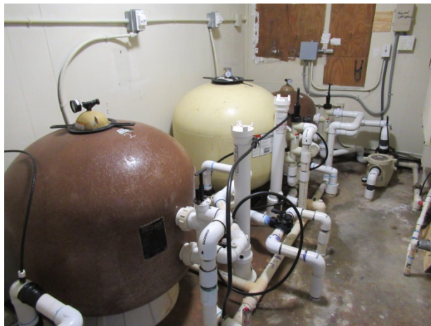
Mechanical equipment overview
