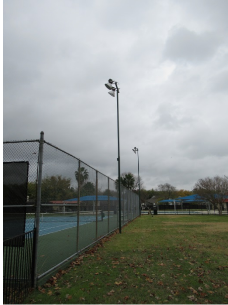
Light pole and fixture
