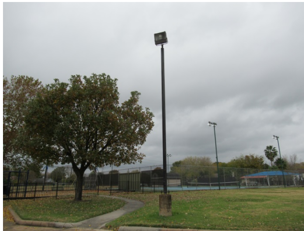
Light pole and fixture
